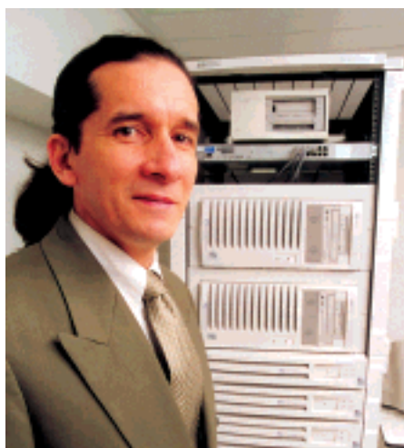
Johnny Trujillo at the remote disaster recovery site.
